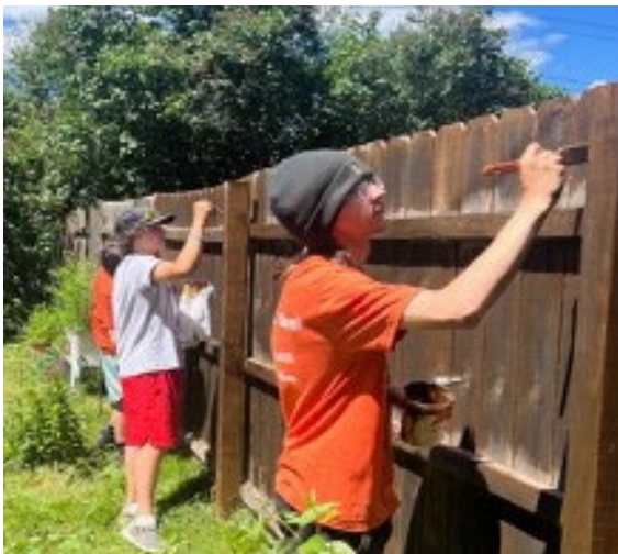
Photos, beginning above right: Youthbuilders help low-income residents repair a deck, install a window frame, and stain a large wooden fence.
